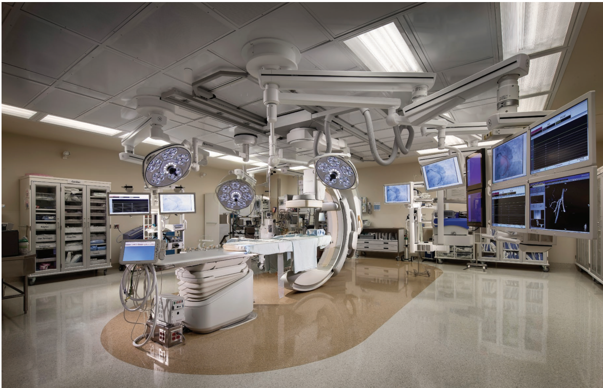
Modern medical illumination: Penn Medicine Lancaster General Health, Hybrid Operating Room (Image source: https://www.ba-inc.com/wp-content/uploads/2014/12/BC_LG_121023_0013_M.jpg )
